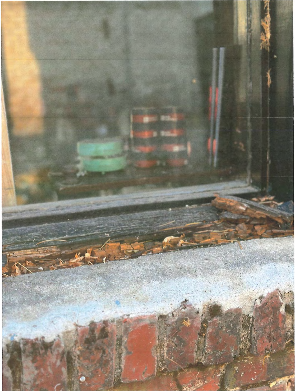
Figure 1.3. Front Window Rotting
