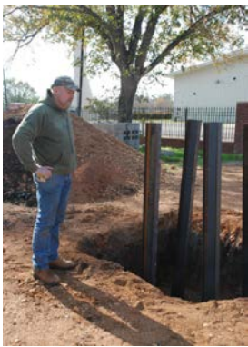
Mayor Mark Bunte surveys the posts that will secure the Angel to the earth.
